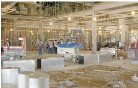
Construction workers break for lunch at the building site for Muskogee Community Hospital on North Main Street. The hospital will be completed next year. Staff photo by Jennifer Lyles
